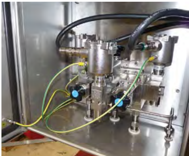
• Actuator control system
